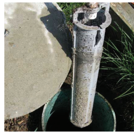
Clogged effluent filters can lead to sewage back ups.
